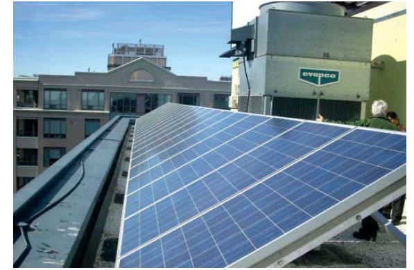
Toronto Community Housing received the Communitas Award in 2011 for leadership in energy management and sustainability. We invest in renewable energy projects, like the installation of solar photovoltaic panels and solar thermal walls, to make our communities greener, decrease our annual energy costs, and help to reduce the city’s carbon footprint.
